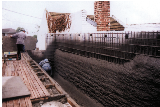
As in this second floor swimming pool, reliable waterproofing prevents leakage from tanked structures into adjacent usable space
