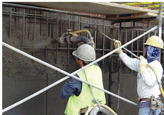
A little advance research will ensure you select the right waterproofing system for your shotcrete structure
