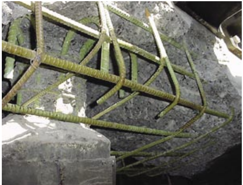
Fig. 1: Impact damage induced spalls in pile cap
