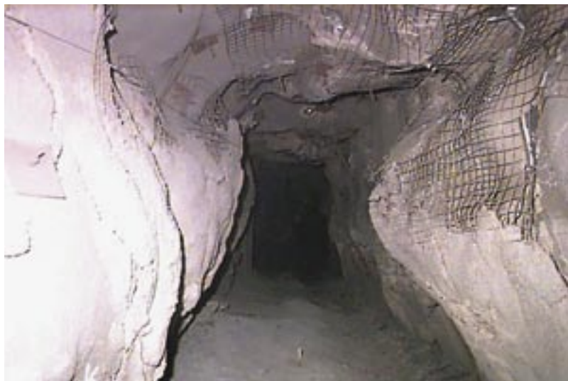
Fig. 2: High deformations are experienced at Perseverance Mine
