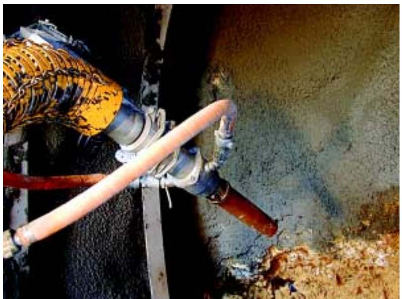
Figure 3, 4, 5 (above): The Aliva AL-500 shotcreting units at the west and east portal headings ready to apply the steel fiber-reinforced, wet-mix shotcrete (left and right) with a closeup inset of the nozzle fixture.
