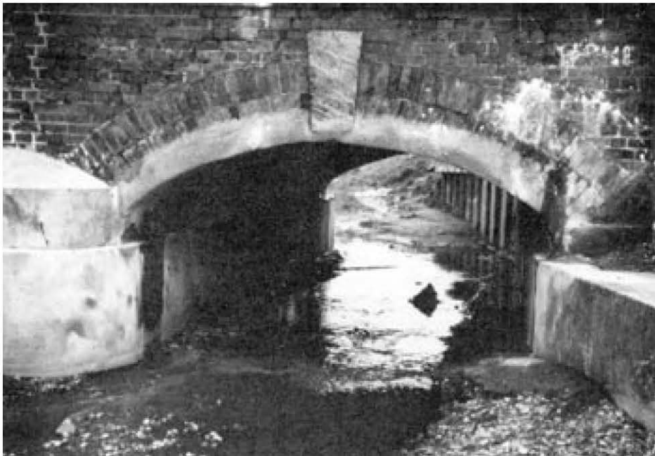
Fig. 1: Brick railway bridge near Birmingham, England, reinforced with about 6 in. (150 mm) of steel fibrous shotcrete.
