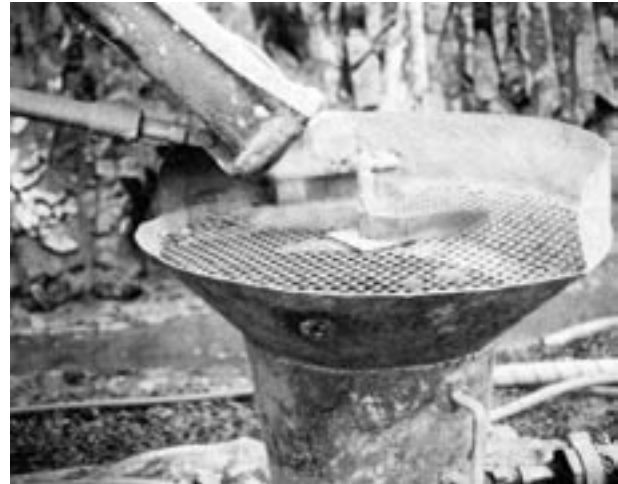
Fig. 3: Modified gun hopper with screen, revolving arms, and pneumatic vibrator.
