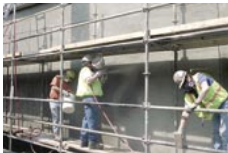
Fig. 10: A polymer-modified cementitious material was applied in two coats to create an aesthetic appearance similar to rubbed concrete.
