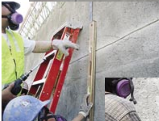
Fig. 7: Aulson crews use a level and straight-edge to ensure vertical alignment in the extremely dense shotcrete surface before saw-cutting expansion joints every 70 ft with a diamond blade.
