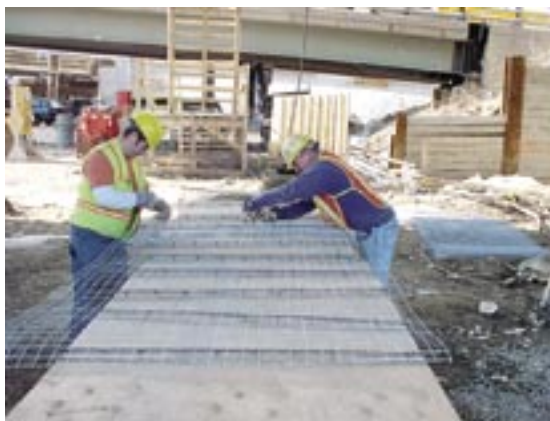
Fig. 4: Wire mesh is attached to epoxy-coated bolster bars with epoxy-coated chairs and vinyl coated wire ties, in preparation for attachment to EPS block.
