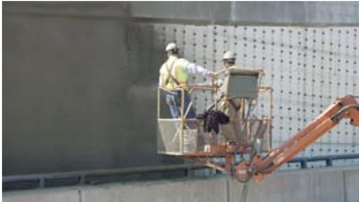
Fig. 6 (above): Aulson ACI certified nozzlemen apply 2 in. of shotcrete at a rate of 400 ft per s over EPS block.
