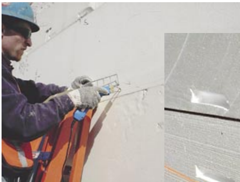
Fig. 2: 1.5 x 1.75 in. recessed notches are etched into EPS with heat-welding gun every 12 in., in preparation for shotcrete adhesion.
