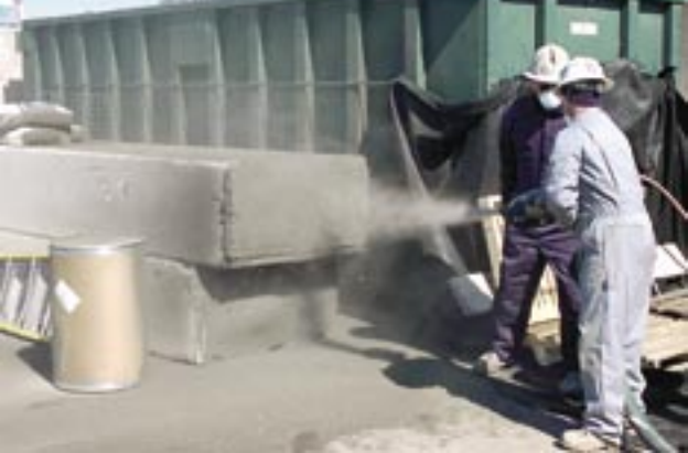
Fig. 1: Aulson ACI certified nozzlemen apply shotcrete to 4 ft test panels of EPS and wire mesh attached with bolster bars.
