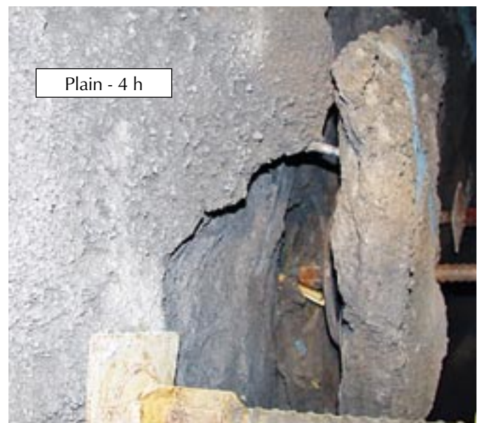
Figure 7: Brittle failure (does not carry load beyond flexural capacity).
