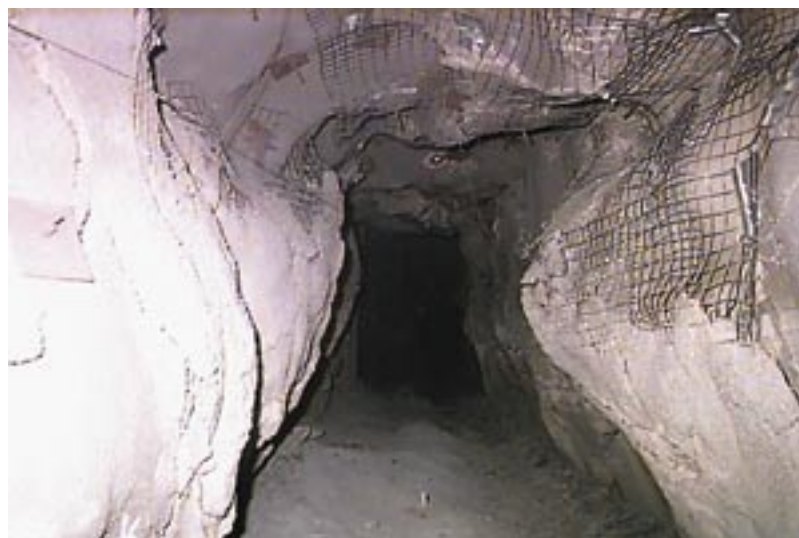
Fiber-reinforced shotcrete has helped to control deforming ground that might not otherwise be minable.
