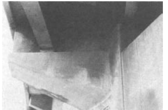
Figure 12: Same cantilevered beam as shown in Fig. 11. The repair has been completed using the shotcrete process.
