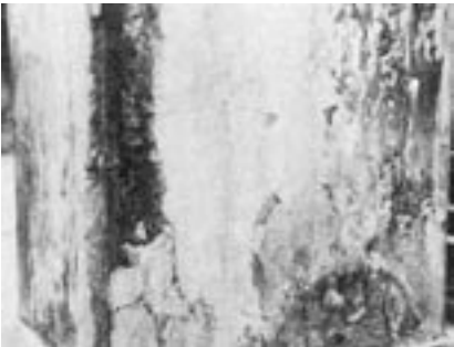
Figure 4: Questionable quality of concrete with scaly finish and reinforcing bars too close to the surface. Reinforcing has developed heavy scale and lost considerable section.
