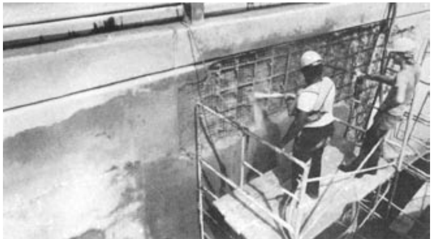
Figure 19: Wetting down an area prior to shotcreting with air-water blast. This procedure cuts down the absorption of mix and water and cleans the area prior to shotcreting.
