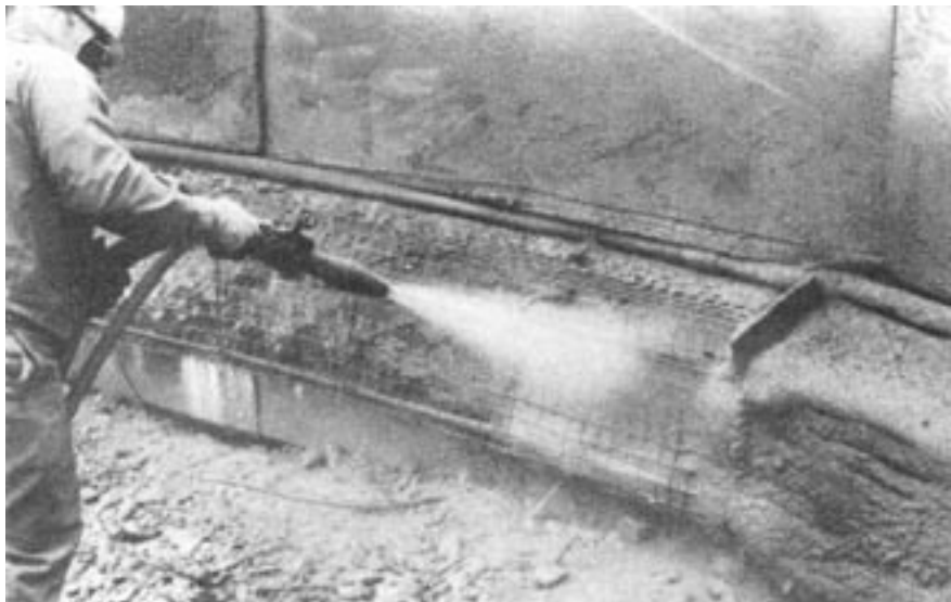
Figure 21: Shotcreting fascia beam. Area to right is over shot. Material will be wasted when surface is trimmed to wire fabric.
