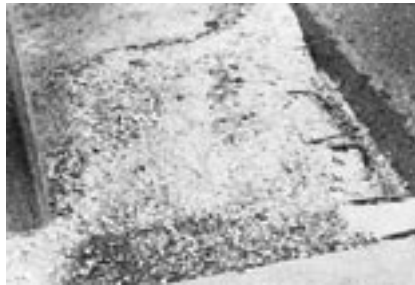
Figure 1: Deterioration of a bridge sidewalk due to freeze-thaw action coupled with liberal use of deicing salts.
