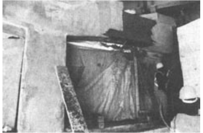
Figure 10: Same general view as Fig. 9. Areas have been shotcreted, finished, and a membrane curing compound applied.
