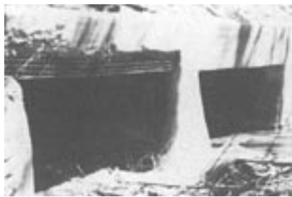
Figure 25: Culvert from Fig. 6 partially restored with shotcrete. Finish is "natural" or "gun finish." Stone wingwall to right has been reintegrated with shotcrete.
