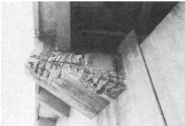
Figure 11: Cantilever reinforced concrete beam support prior to repair. Note penetration of rust to areas adjacent to reinforcing.
