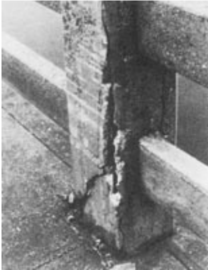
Figure 3: Crack development in handrail post-penetration of moisture to the reinforcing with the subsequent rusting, cause the concrete to spall and break away.
