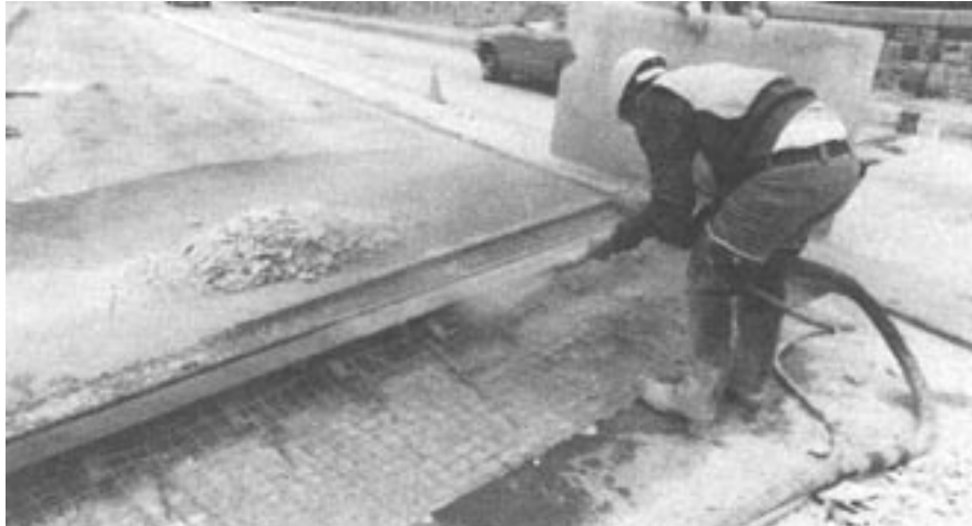
Figure 20: Shotcreting expansion dam that had become loose and had to be rewelded. Care must be taken by nozzleman to see that rebound does not build up in the inaccessible areas.
