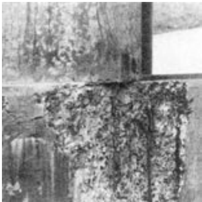
Figure 13: The deterioration of the concrete in this crash barrier and column base is primarily due to roadway splash adhering to the surface and going through many freeze-thaw cycles. Deicers accelerated the process.
