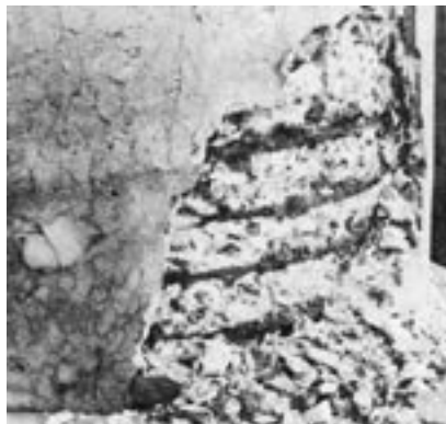
Figure 2: Crack development of column base followed by rusting of the reinforcing steel causing aggravated decay of the concrete. Water and salt leaking from bridge deck plus freezing splash water from the roadway have combined to cause this distress.
