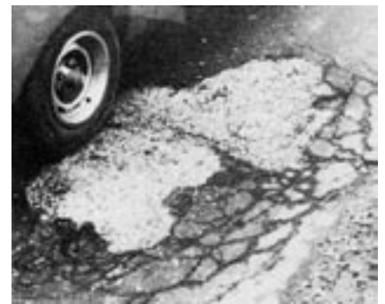
Figure 7: Bituminous surface breaking up exposing deck to corrosive influences. Even though surfacing has been patched, concrete underneath is severely deteriorated and ready to break through. Area in lower right hand corner is rubble from sidewalk deterioration.
