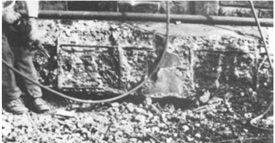
Figure 16: Same fascia beam as shown in Fig. 14. Chipping concrete with a pneumatic chipping hammer. The concrete is soft, spongy, weak, and relatively easy to remove. Chipping must continue until a hard surface is exposed.
