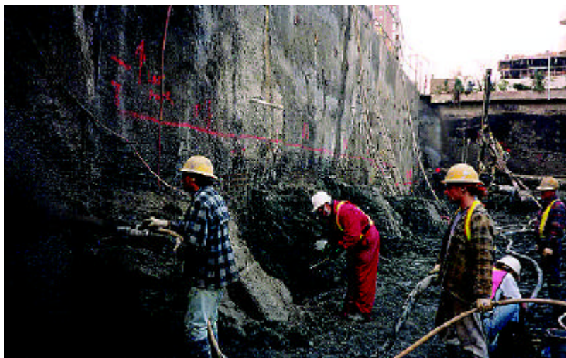
Figure 1: Application of shotcrete for support of stressed tie-back construction excavation in Vancouver, B.C.
