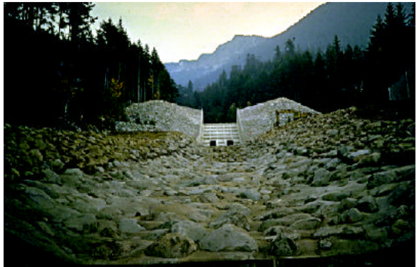
Figure 4: Use of shotcrete for erosion control at Harvey Creek, Lions Bay, B.C.
