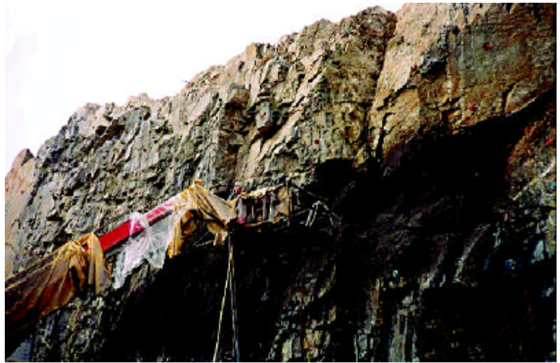
Figure 3: Shotcrete application for rock slope stabilization at Stave Falls Hydroelectric Project, Mission, B.C.
