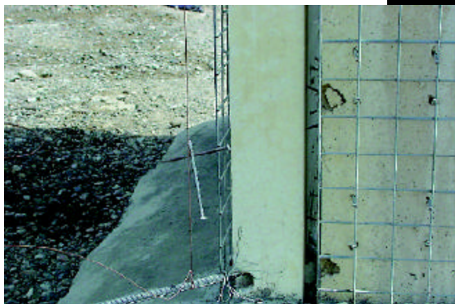
Figure 3: Use of a guide line to make the corner shown in Figure 1.
