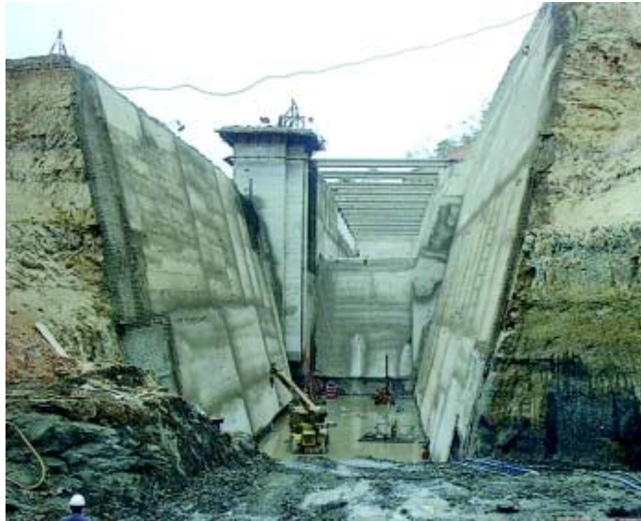
View through the spillway of the Conguillo Dam, showing shotcrete directly onto the excavation.
