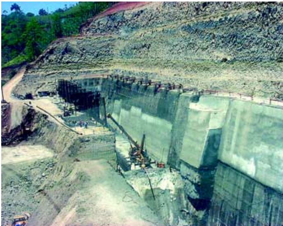
Note the heavy rebar cages on the left, which are prepared to receive shotcrete.
