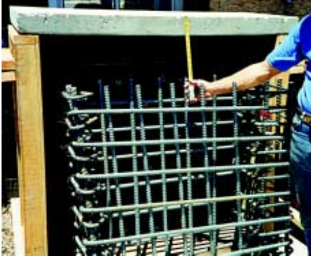
(above) "Worst-case" simulation test panel for Stanford University project incorporated a simulated concrete soffit. (right) Completed in-fill section of wall.
