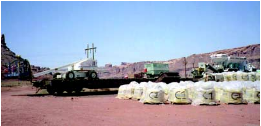
Figure 4: Sling bags of shotcrete mixture and work train at a railroad siding.
