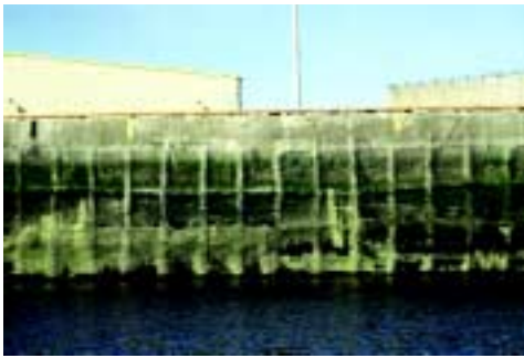
Figure 7: View of shotcreting in 1995, after 10 years of service with buildup of shotcrete at reinforcing steel to help alleviate restrained drying shrinkage cracks.
