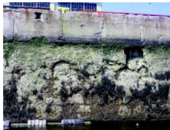
Figure 2: Deterioration in intertidal zone of berth face.
