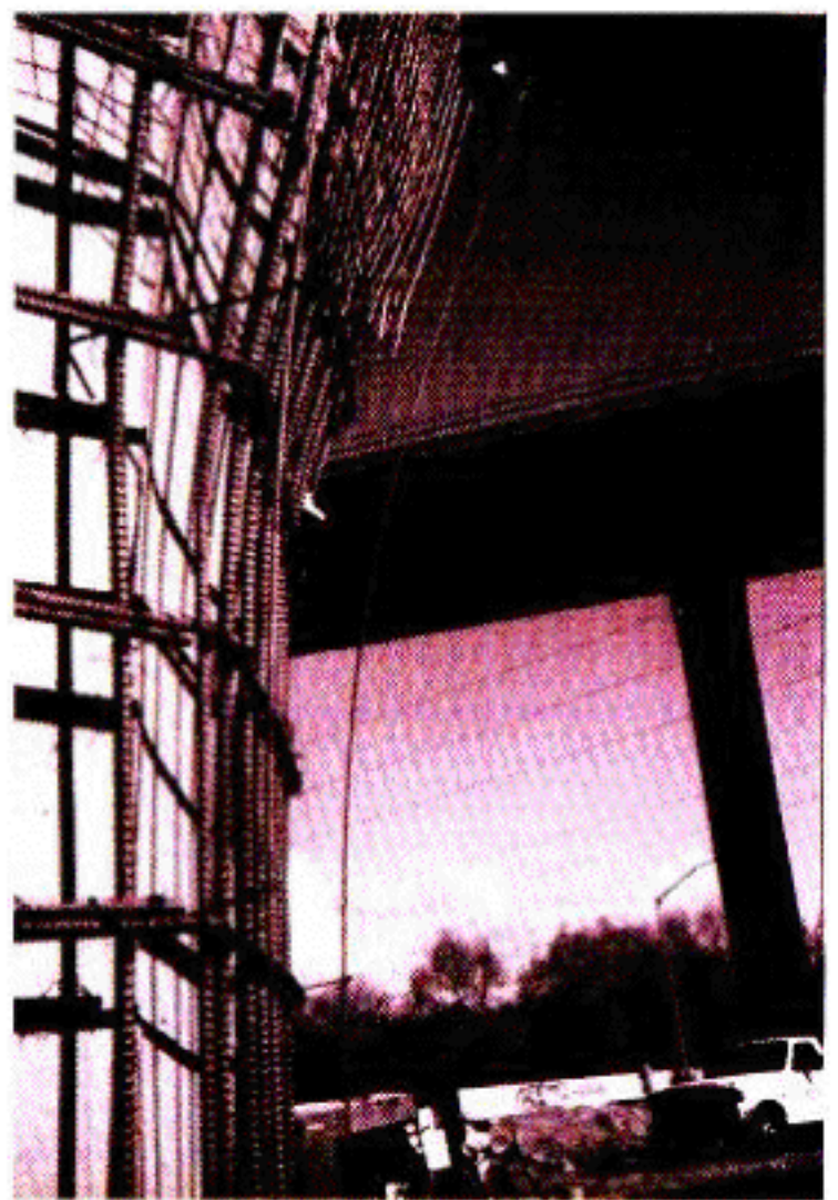
Figure 3: Small diameter steel rod delineates final curvature contour of a bridge pier.
