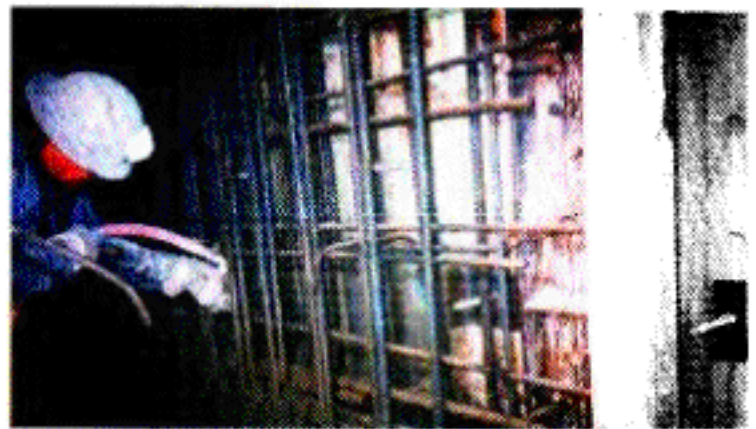
Figure 1: With the wet mix process, the nozzle can be discretely directed into and through the reinforcing.
