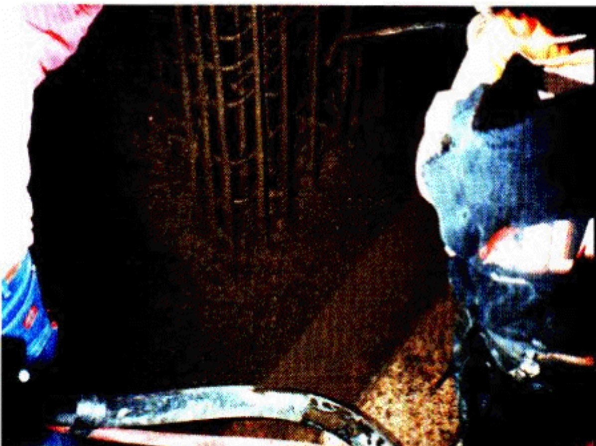
Figure 6: Use of a blowpipe constantly following the nozzle operator is essential to prevent rebound accumulation in heavily reinforced work.
