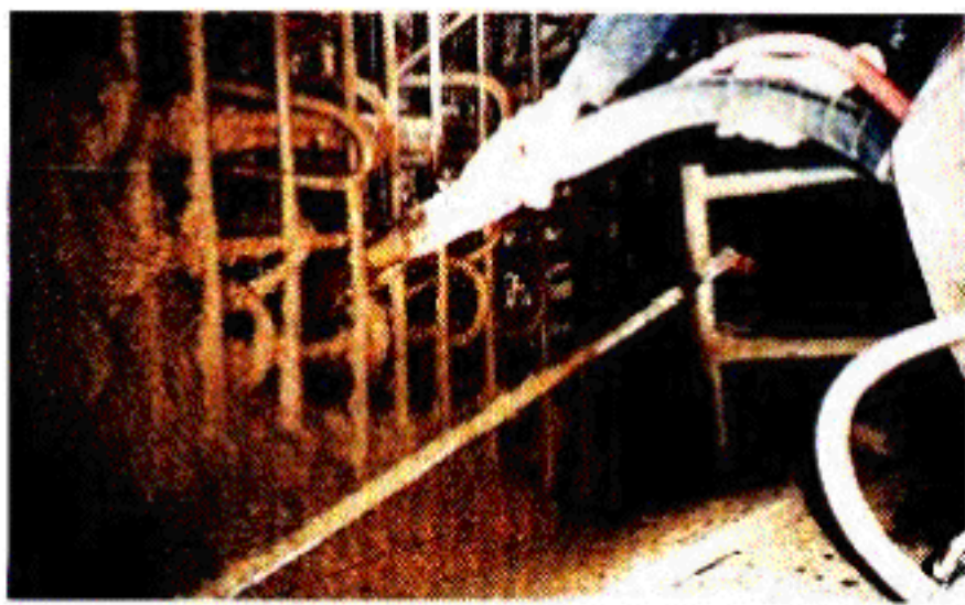
Figure 4: Nozzle is actually pushed into the reinforcing in order to completely fill this thick, heavily reinforced section.
