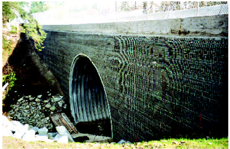
Figure 1. North face of MSE wall before repairs.
