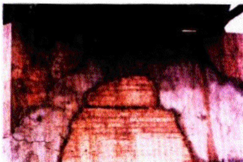
Figure 6. Bridge pier repaired with an accelerated, steel-fiber-reinforced shotcrete with drying shrinkage cracking.
