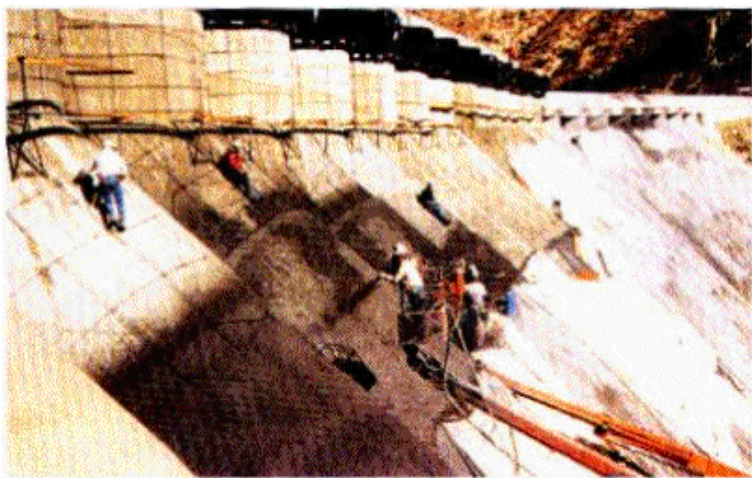
Figure 7. Littlerock Dam seismic retrofit with crack-free, wet-mix, steel-fiber-reinforced silica fume shotcrete. Note: curing blankets.
