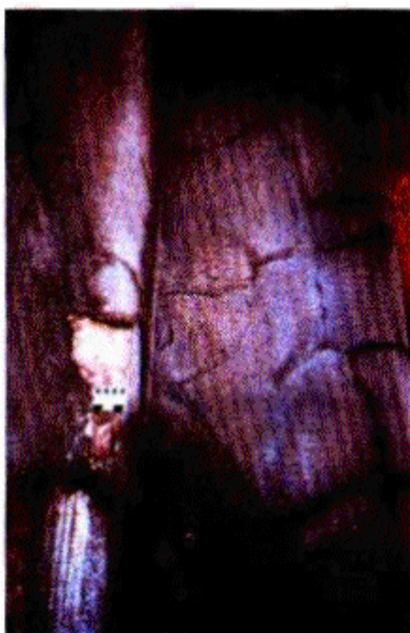
Fig. 1: Edge curling and delamination in a shotcrete-repaired bridge pier with improper surface preparation.
