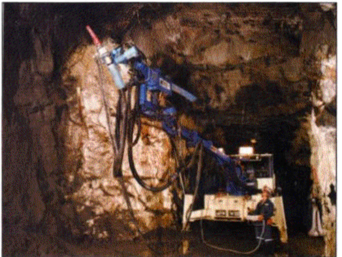
Figure 4. Computerized, robotic, spraymobile; capable of laser profiling of heading to be sprayed and subsequent computer control of spraying operation.
