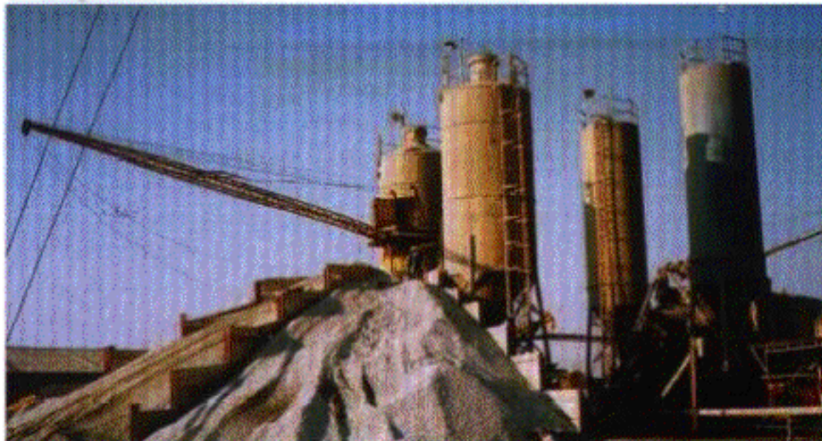
Figure 1. Surface batch plant.
