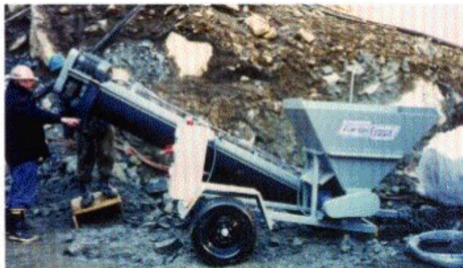
Figure 5. Picture of a pre-moisturizer machine used to lower dust emission underground.
