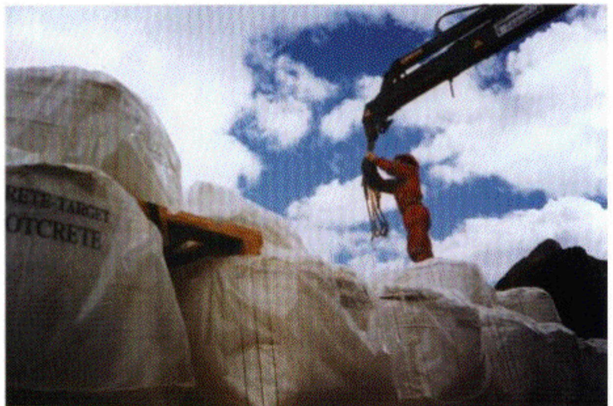
Figure 3. Worker unloading bulk bags of shotcrete ready to be used at Antamina Mine.
