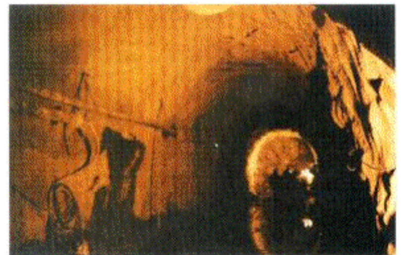
Figure 4. Shotcreted tunnel and inlet face with type III ground to be supported with shotcrete.
