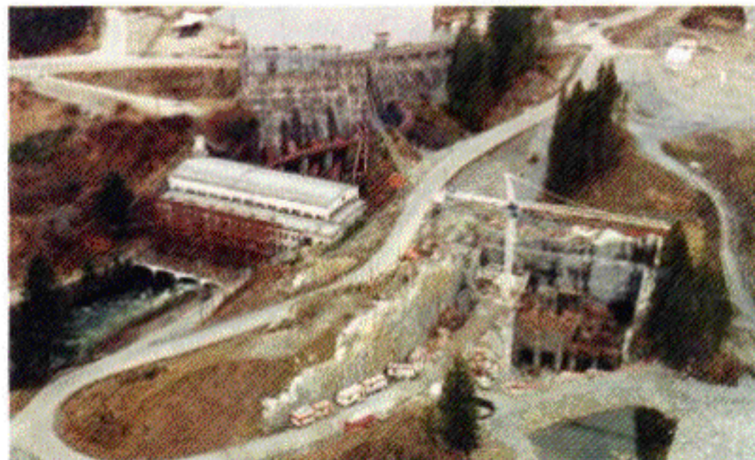
Photo 1. Existing Stave Falls power house on left with new tunnel construction on right.
