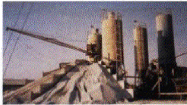
Photo 1. Surface batch plant.
