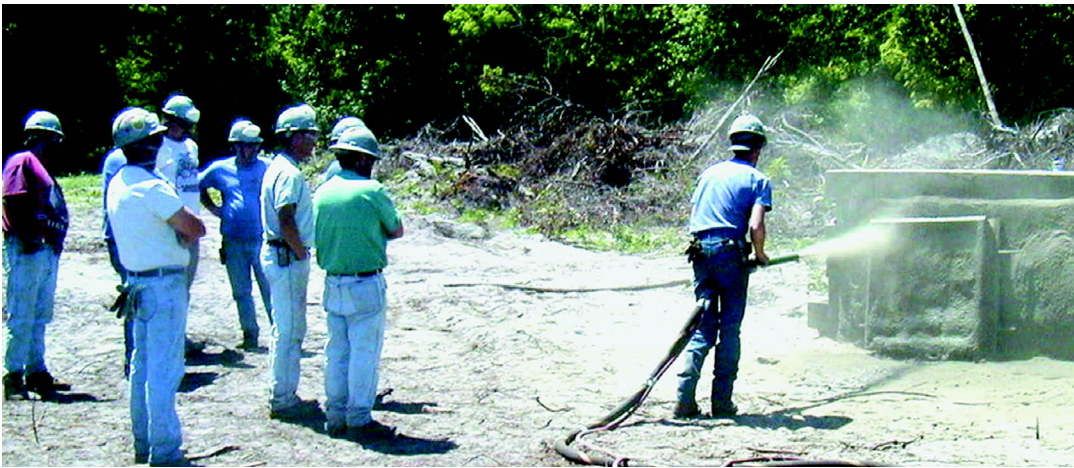
Figure 2. Shotcrete nozzleman shooting a test panel in an ASA-sponsored Nozzleman Certification Program.
