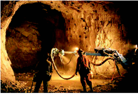
Figure 4. Application of wet-mix shotcrete in a tunnel using a remote-control application boom (provided by MBT Shotcrete and Underground Group).
