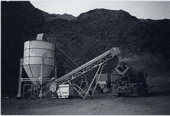
Figure 5. Bulk shotcrete mix being loaded from a silo to a mixer truck in Chile.
