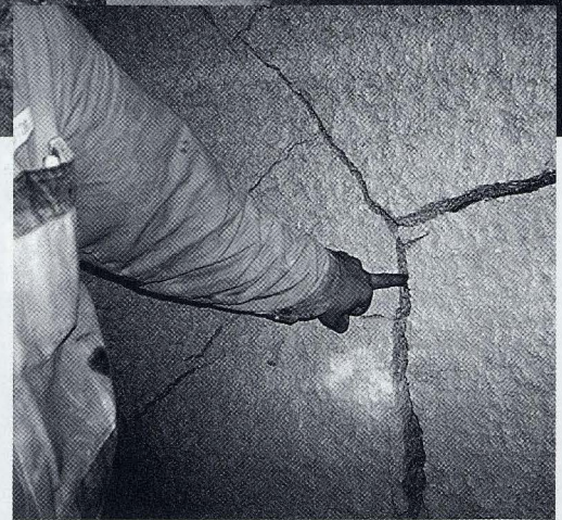
Figure 2. Damage to shotcrete due to blasting stresses in a Canadian mine.
