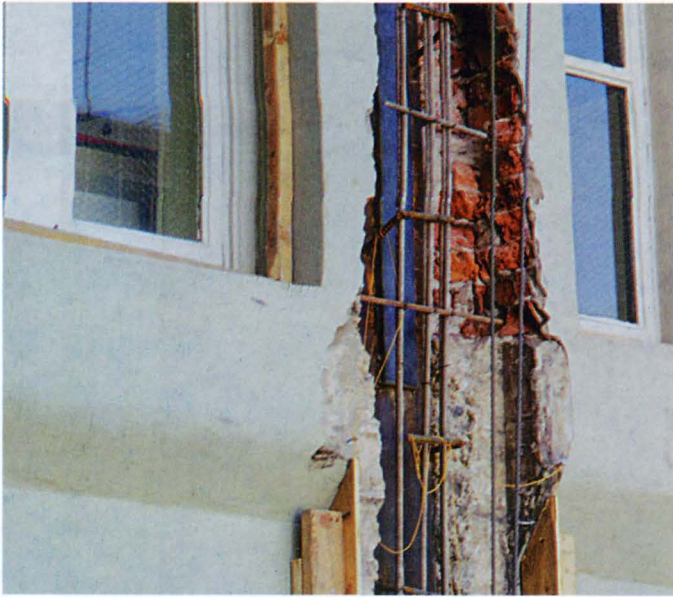
Figure 4: View of a prepared column ready for shotcrete application. Note installed new steel plate and rebar.
