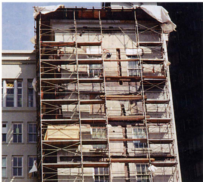
Figure 3. Installed scaffolding and removal of brick masonry on a column line on South face of building
