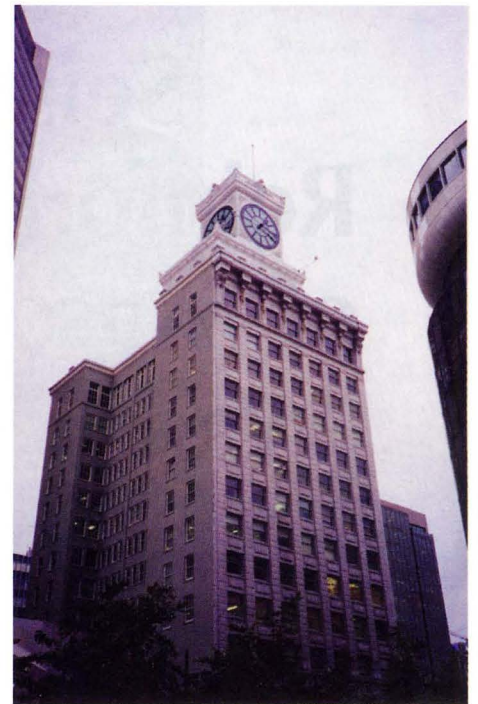
Figure 8: View of north and west faces of Vancouver Block building after completion of shotcrete repairs and application of an elastomeric coating.
