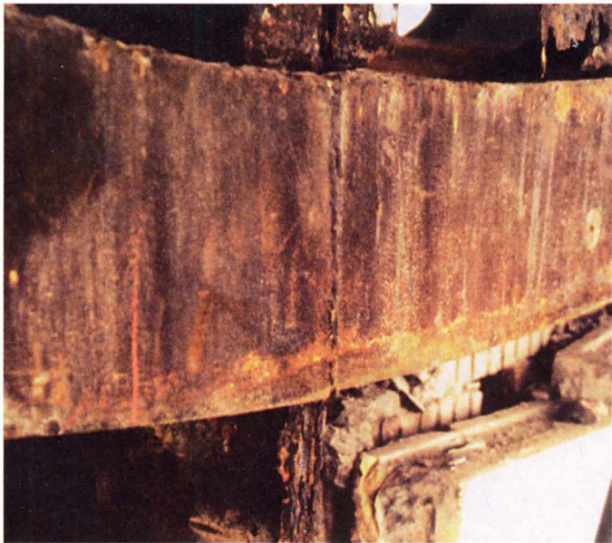
Figure 2. View of corrosion in a steel column prior to repair.
