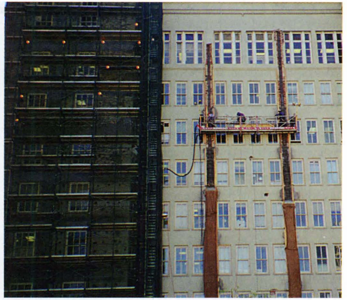
Figure 5: Remedial work being conducted from a swing stage on north face of building. Note burlap wet cure of completed shotcrete repair.
