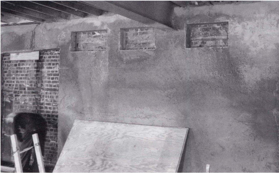
Incorporation of shotcrete shear walls made it possible to include this historic structure into a modern federal courthouse complex
